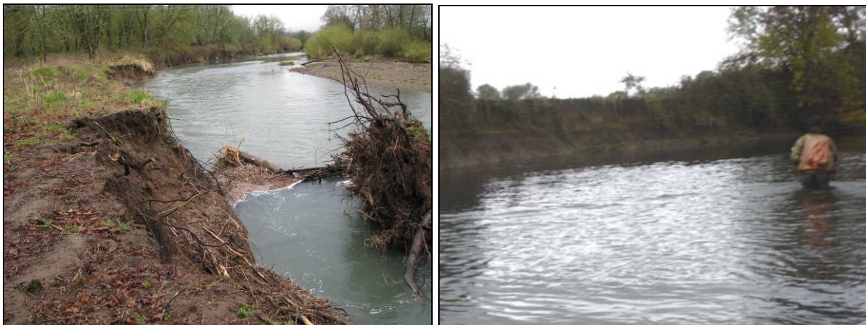
Figure 4-13. Example streambank failures in Reach 4 include the Smith property (left – photo courtesy of T. Putney) and the bank at Sta. 354+00 (right).
