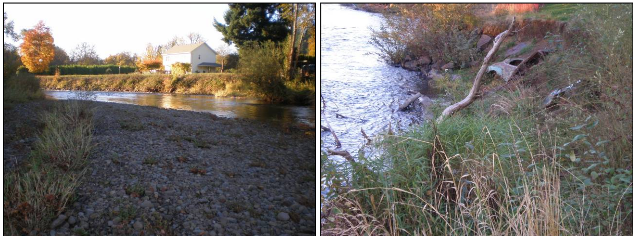
Figure 4-5. Bank stabilization sites in Reach 2 include the house protection at Sta. 160+00 (left) and at Pioneer Park.
