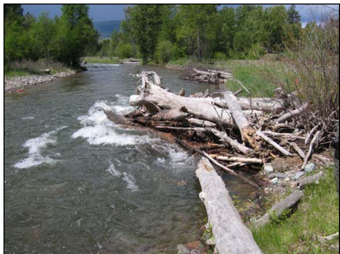
Figure 5-2. An ELJ constructed on the Jocko River in western Montana following two run-off events.
