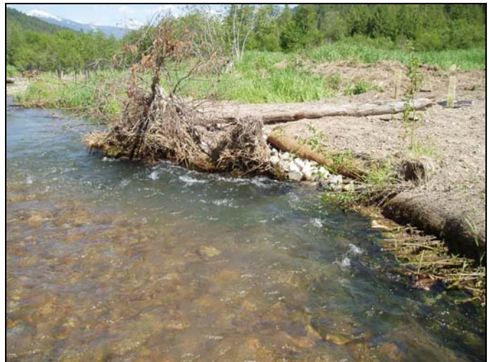
Figure 5-4. A large wood habitat composite with adjacent soil lift on Pilgrim Creek in western Montana.
