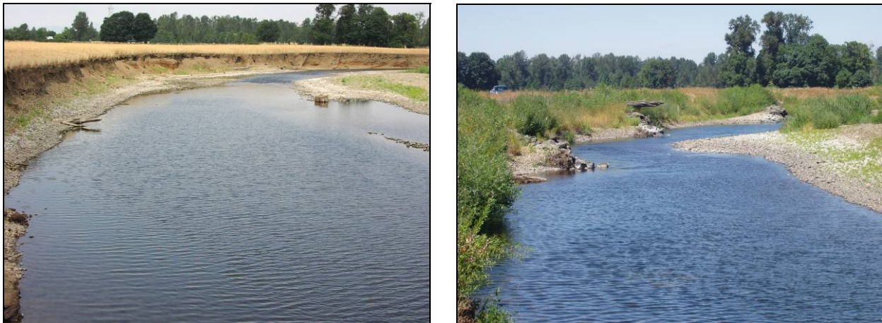
Figure 4-1. Examples of eroding bank (left) at the Carbajal site pre-project and more recent (right) photo showing effects of bank stabilization using rock barbs and revegetation.
