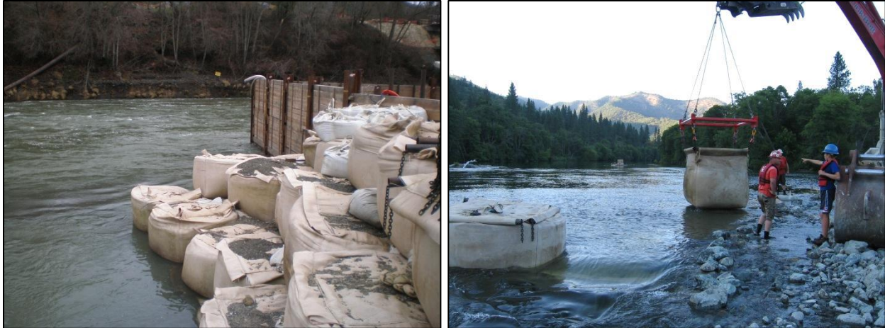
Figure 4-5. Example of stacked bulk bags used to isolate a work area on the Rogue River at the Savage Rapids Dam Removal project (left). A bulk bag being moved into place as part of the Gold Hill Dam Removal project (right).
