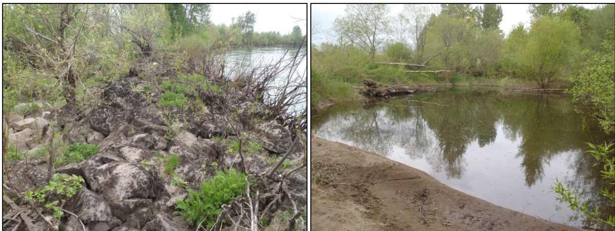
Figure 4-2. An upstream view of the Coon Creek revetment located on the river-right bank of the Willamette River to the west of BRSP (left). A pond located between the revetment and gravel pit pond (right).
