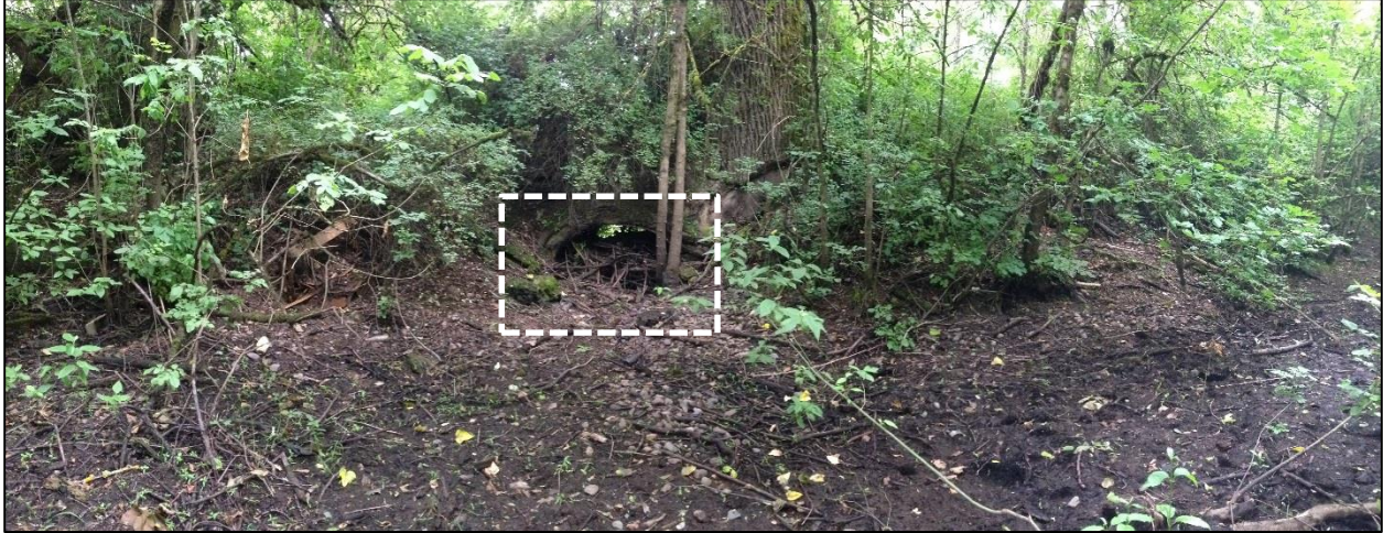
Figure 4-7. An upstream view of the culvert (white box) at ES-1. The mature cottonwood is located to the right of the culvert.
