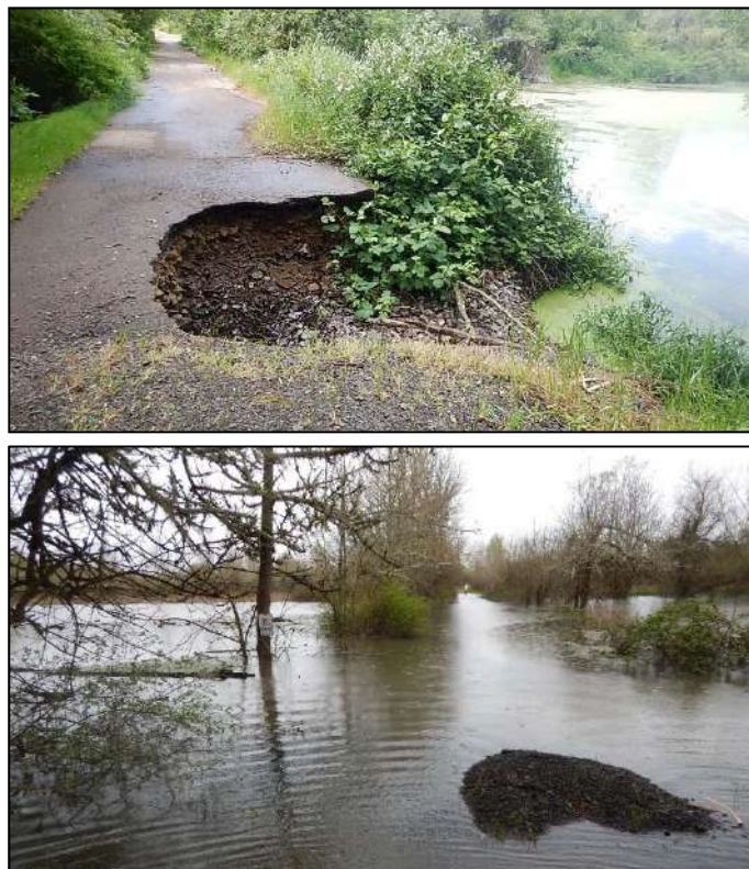
Figure 1-3. Similar view of the OPRD road during low (top) and high (bottom) flows on Dead River. The bottom photo was taken at approximately 30,000 cfs at the Albany gage on the Willamette River downstream of the Dead River confluence with the Willamette River. The gravel deposit in the lower photo is adjacent to the failure culvert.
