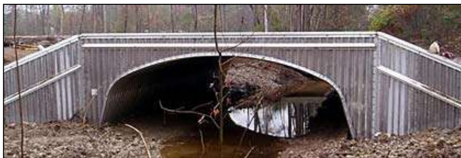
Figure 6-6. View of an aluminum structural plate box culvert.
