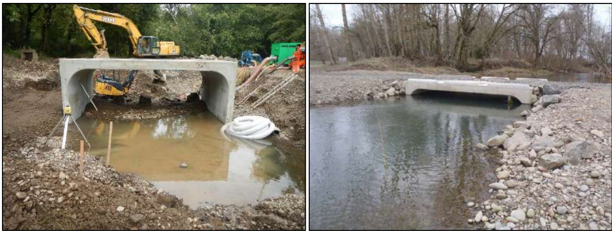
Figure 6-2. Installation of the Green Island box culvert in 2013 (left) and post-high water in 2014 (right).
